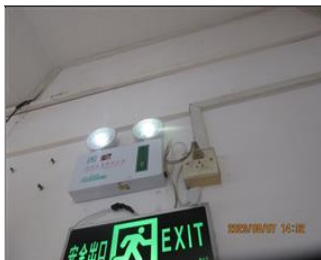
Photo of fire safety equipment emergency light test.JPG
