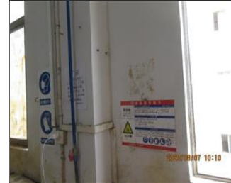
Photo of the personal protection equipments (if applicable) PPE warning sign.JPG
