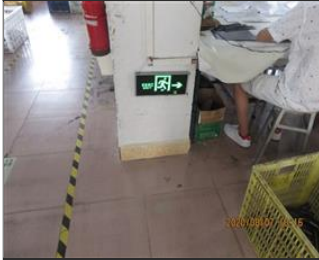
Photo of fire safety equipment evacuation sign.JPG
