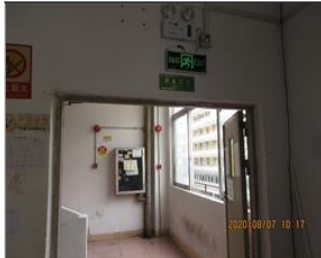
Photo of fire safety equipment emergency exit.JPG
